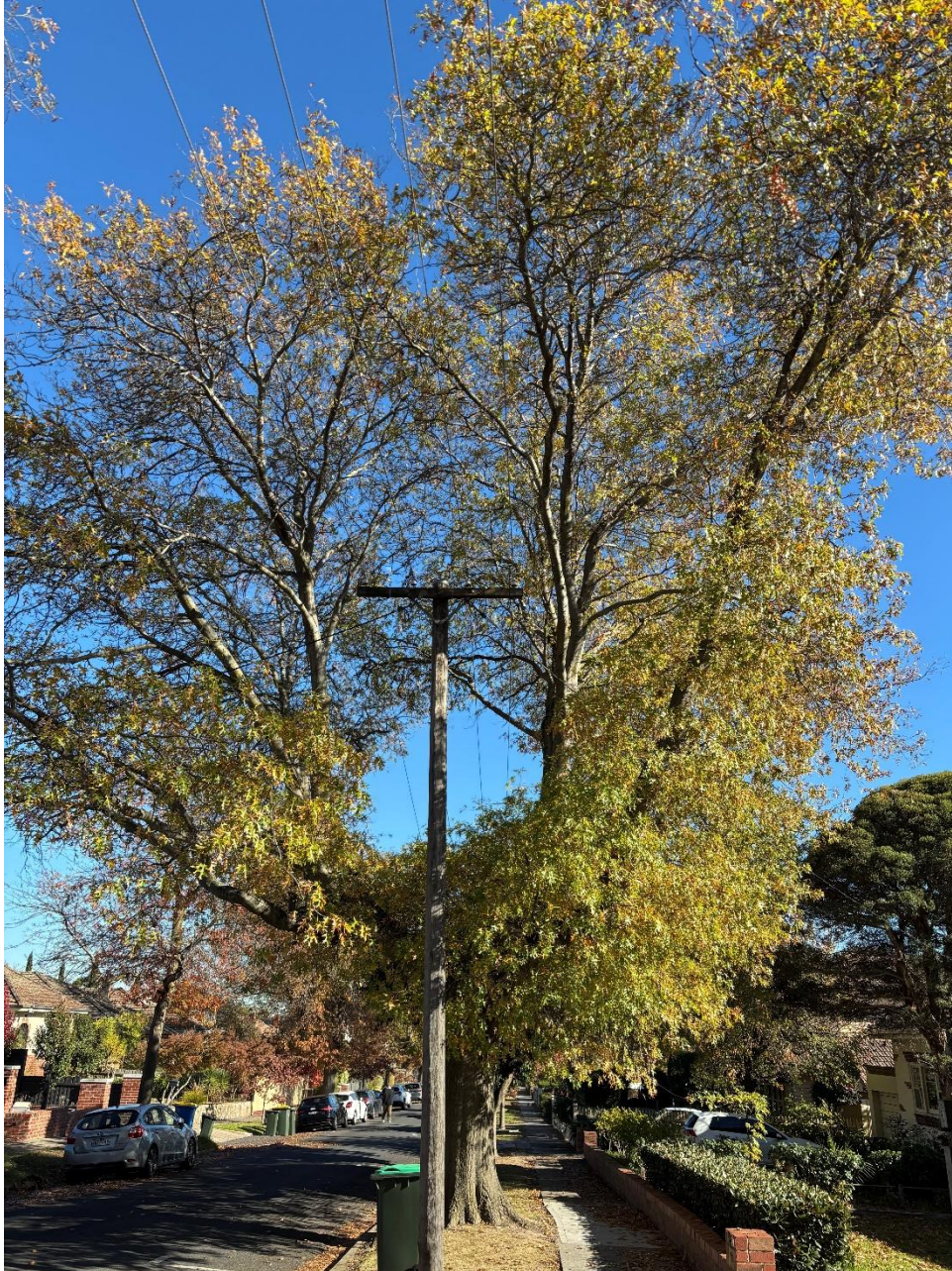
A street tree successfully managed in Boroondara with branches 30cm from uninsulated LV lines
